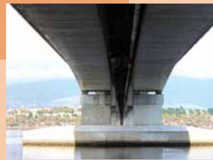
The pipeline beneath the Bowen Bridge.
